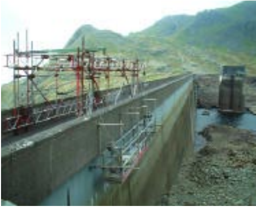
Access platform suspended from special mobile rig on the dam crest for second round of coating trials
